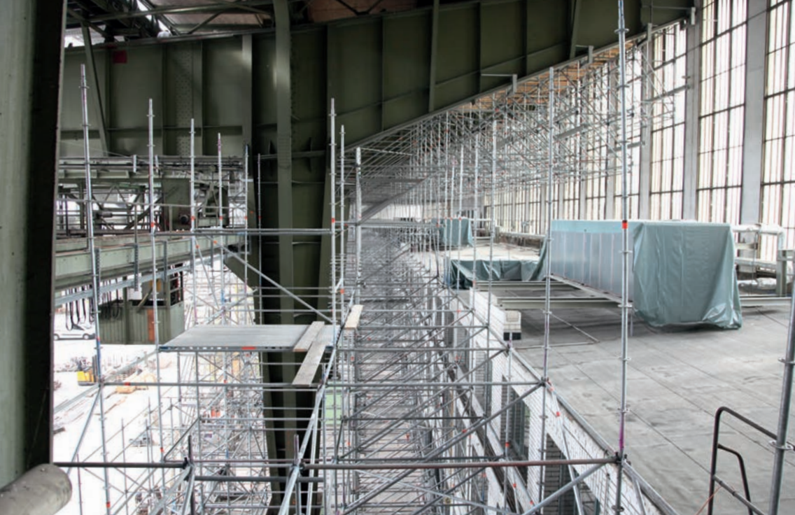
Layher Allround Scaffolding was used for the shoring structure in front of the interior building sections and it supports the front section of the work platforms below the ceiling.
