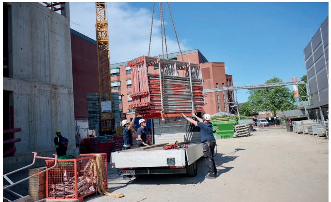
At the construction site, Layher logistics solutions demonstrate their tried and tested efficiency.
