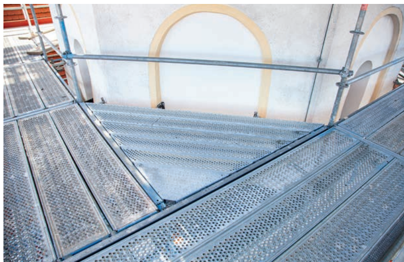
The scaffolding corners resulting from the architectural geometry are covered securely by U-steel decks 45°.
