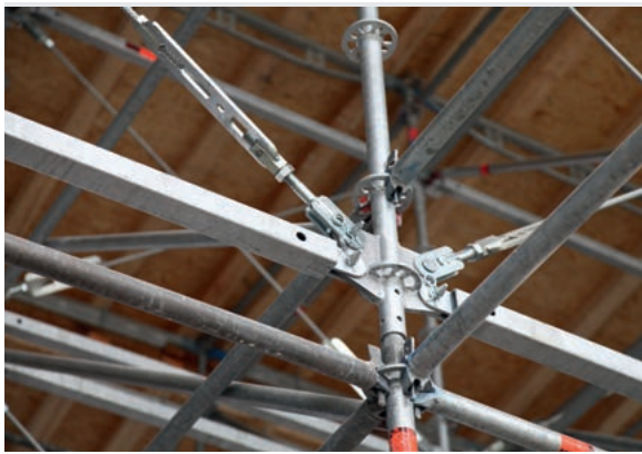
The Layher Allround FW System is at the heart of the entire structure.
