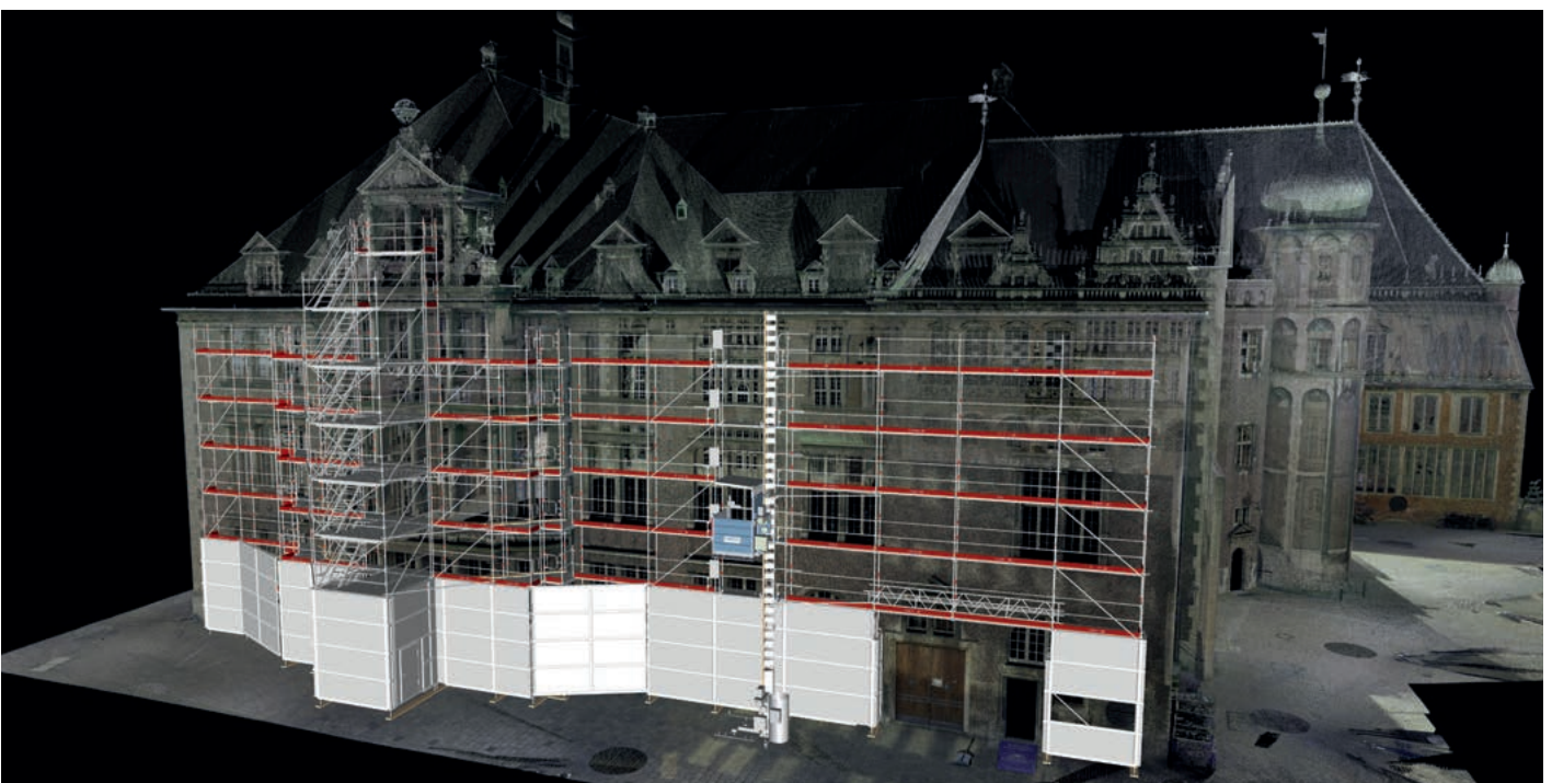
The features of the entire Town Hall were captured in great detail with a 3D laser scan. In the form of a digital twin, this information was applied for reliable scaffolding planning and material logistics at the Bremen city centre.
